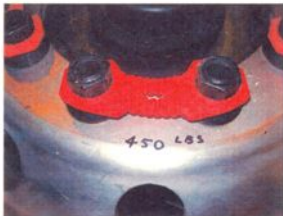
Figure 11 : Sample 10-03-C0152-9 installed on 450 ft-lb torque nuts
