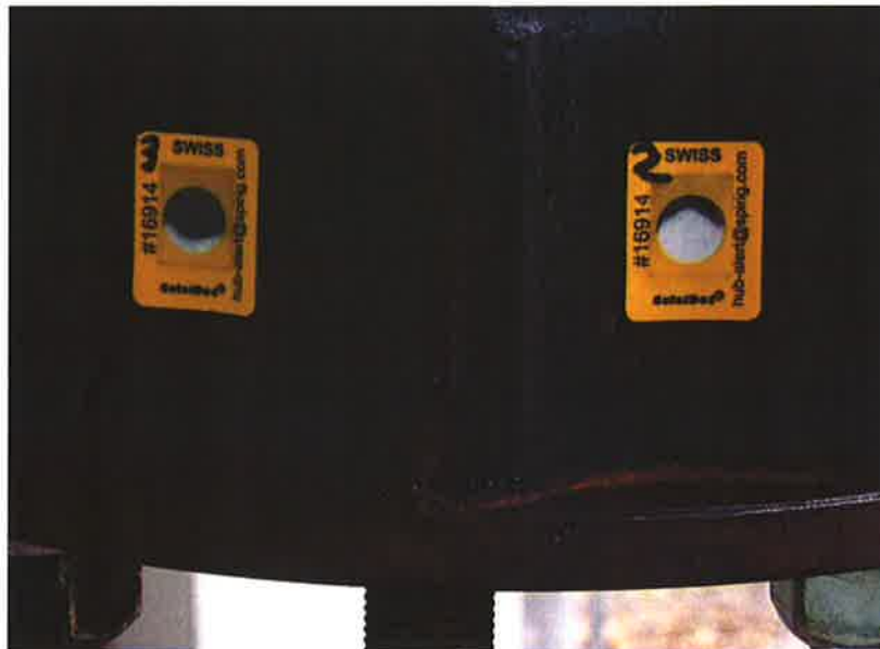
Figure 10A : Steel hub with labels – Partial temperature activation of HUB ALERT™ heat sensing labels (Exova sample numbers 11-15-0165-29 and 30, labels applied to side of hub)
